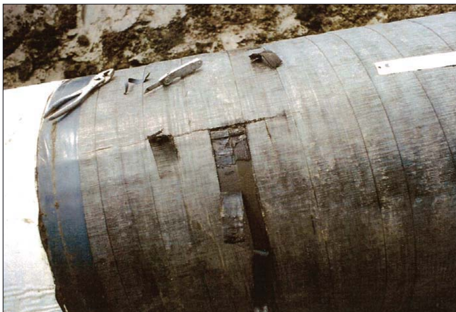
Intentionally applying this geotextile mesh backed coating to a partially wet pipe surface and reexamining it 3 years later found a pH of 11 on the disbonded areas of the pipe, showing continued shielding. The coating did not adhere to the wet parts of the pipe surface but adhered well otherwise (Fig. 3).
