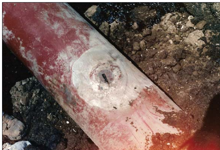
A large boulder sat on top of this 12-in. OD fusion-bonded epoxy coated pipe, shielding CP to it (Fig. 1).
