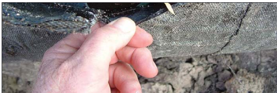
Checking pH under this disbonded geotextile mesh backed coating yielded a measurement of roughly 10, showing the coating's nonshielding properties (Fig. 2).
