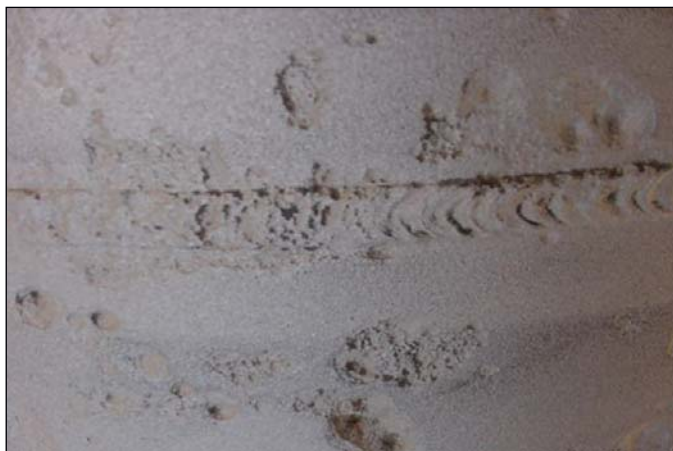
This corrosion, found in 2006, lay under a shrink sleeve applied 9 years earlier. The shrink sleeve shielded the pipe from CP. Pipe potentials met all National Association of Corrosion Engineers criteria (Fig. 4).
